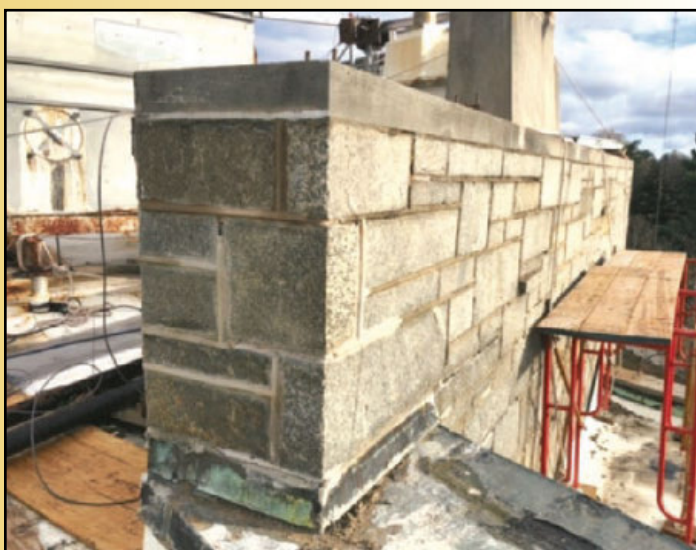
Photo shows the missing mortar joints in the stone wall and the capping. In the part closest to the viewer, the tests for different mortar joint colors and finishes are visible.
